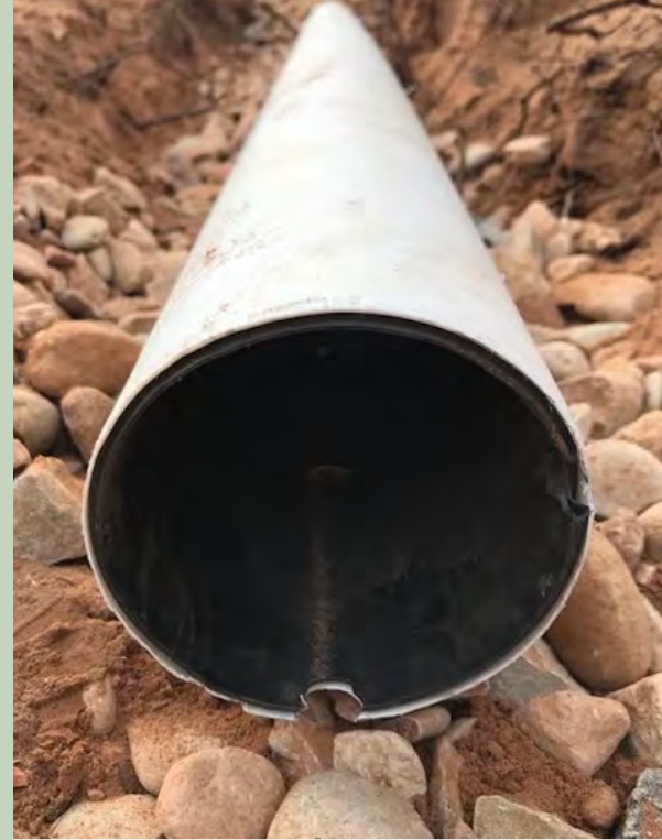
Bronze Drainfield - Zion National Park, UT
